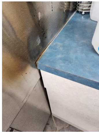
Heat damage due to the burner
